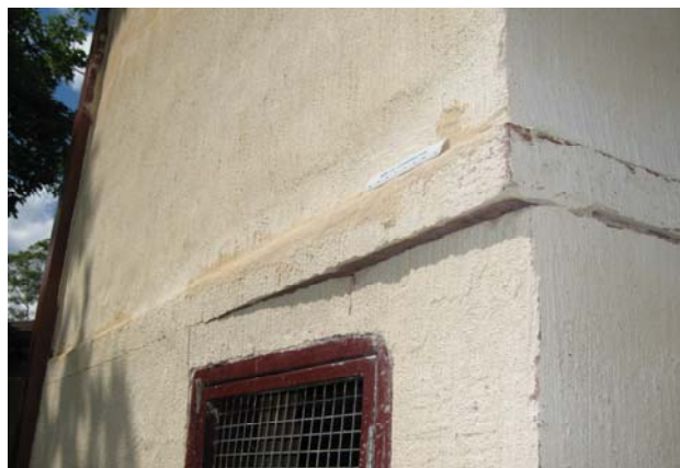
Figure 1 - Structures Affected by Horizontal Shear Deformations
