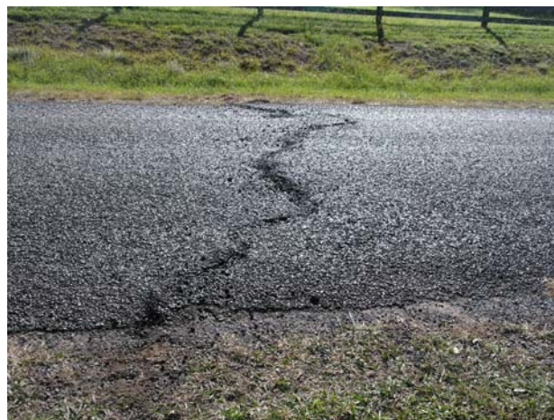
Figure 3 - Mining-induced surface wrinkles
